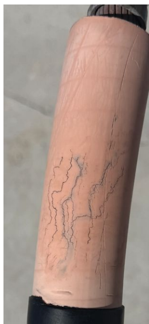
Partial Discharge on a Medium-Voltage Cable
