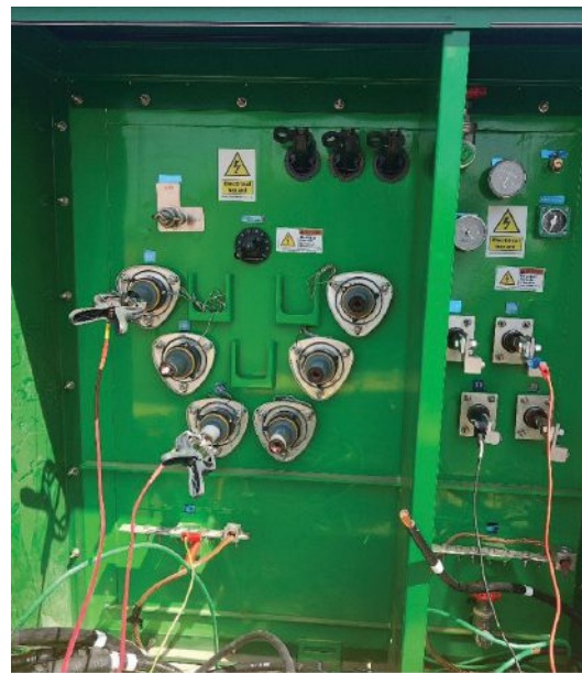
Figure 3: Transformer Turns Ratio (TTR) Testing Connections
