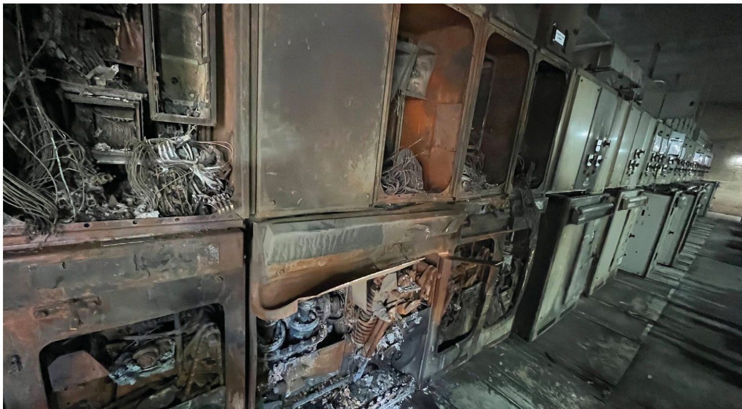
Switchgear Failure Due to Undetected Partial Discharge
