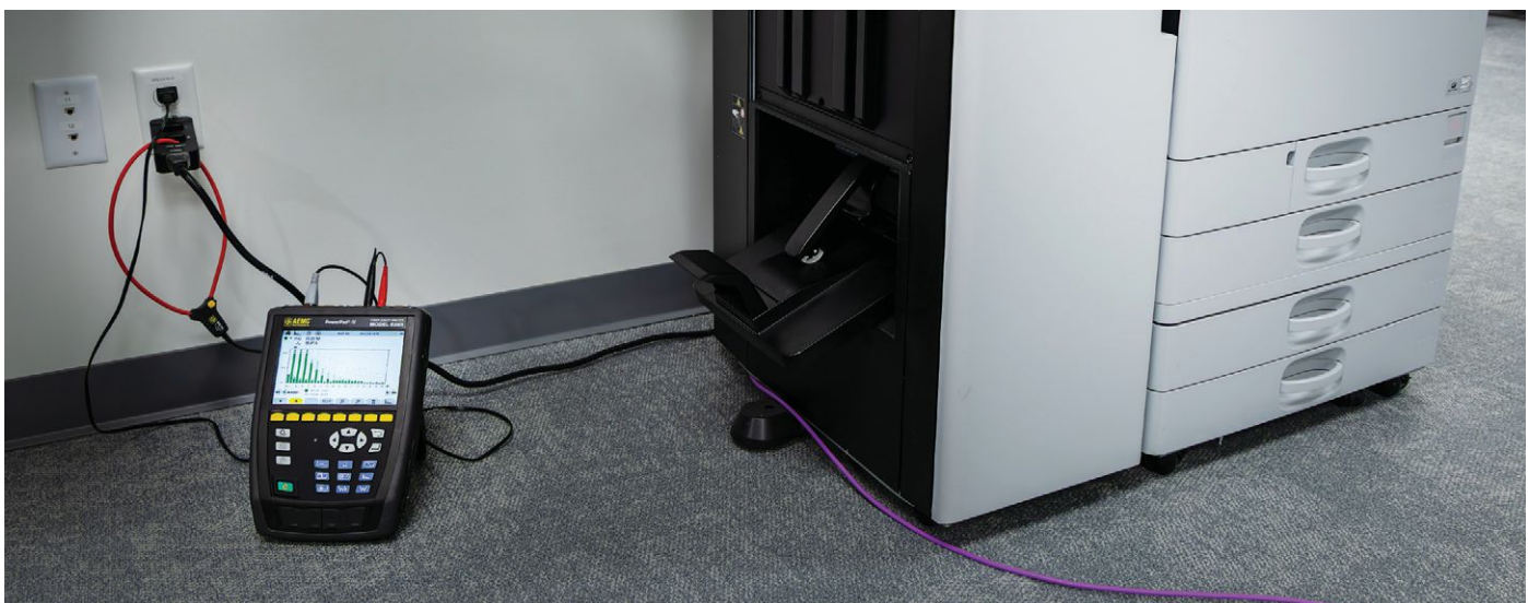
Figure 2: Single-Phase Outlet Power Quality Analysis
