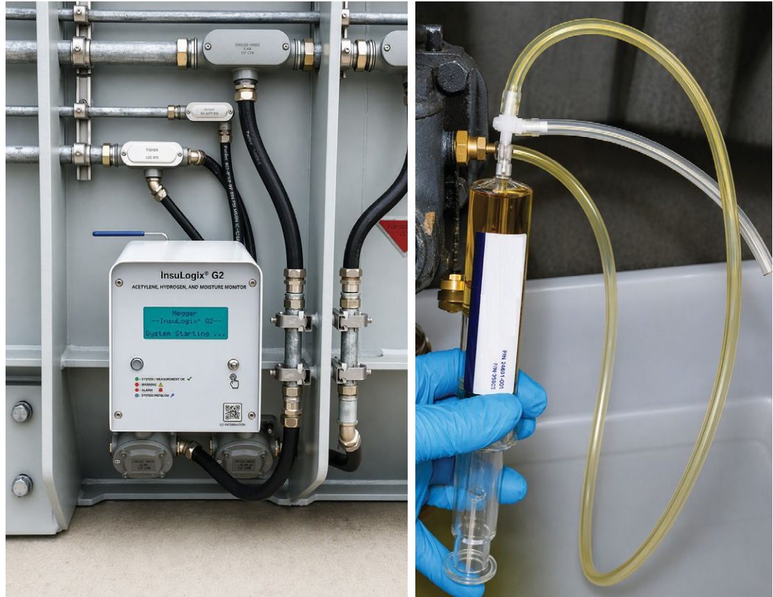
Figure 3: Installed DGA Monitor vs Manual Oil Sampling
