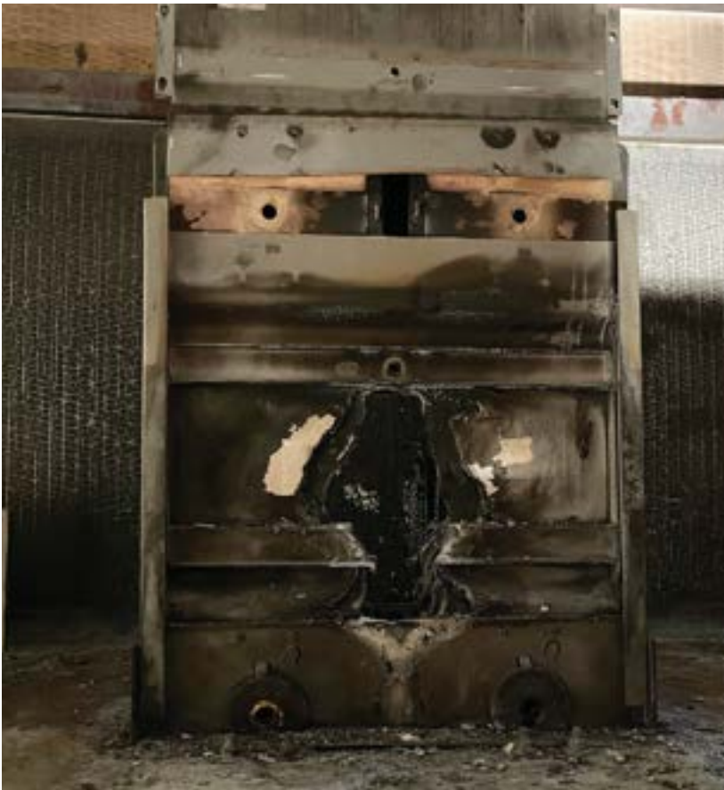
Figure 3: Results of an arc flash in a section of low voltage busway. The root cause was determined to be water ingress.
