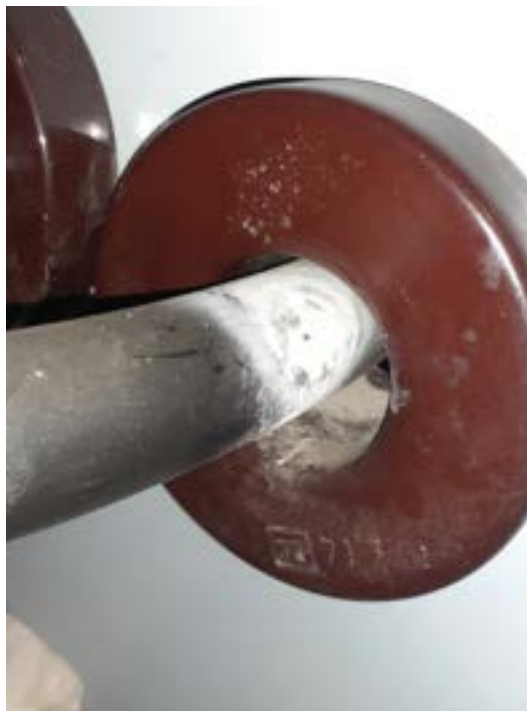
Figure 2: MV Unshielded Cable between Transformer and Switchgear Showing Surface Tracking, Corona Activity, and Degraded Insulation Material
