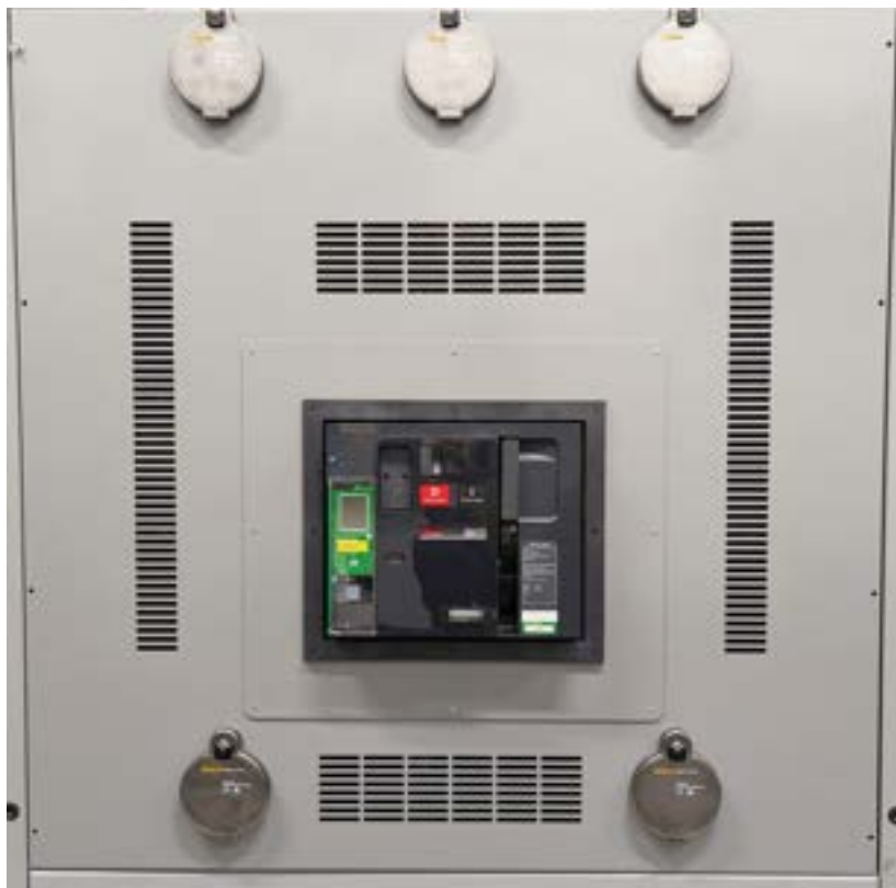
Figure 2: 3,000-A Square D MTZ Replacement Circuit Breaker Retrofit
