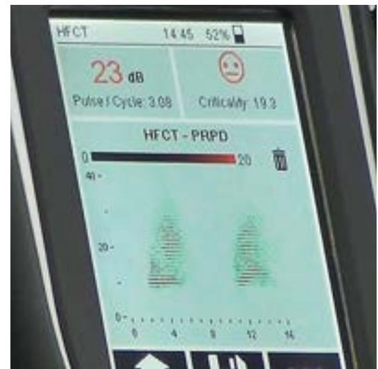
Figure 7: PRPD Patterns Captured with HFCT Confirming a Valid PD Defect
