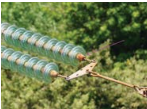
Figure 1: RGB Imaging — Insulator Corrosion
