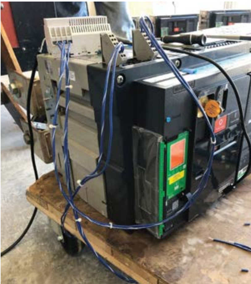
Figure 8: MTZ Breaker Power Supply Connections for ERMS Defeat PHOTO COURTESY JESSE MASSMAN
