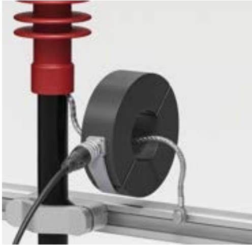
Figure 5: HFCT Clamped on the Cable Termination at the Grounded Cable Gland
