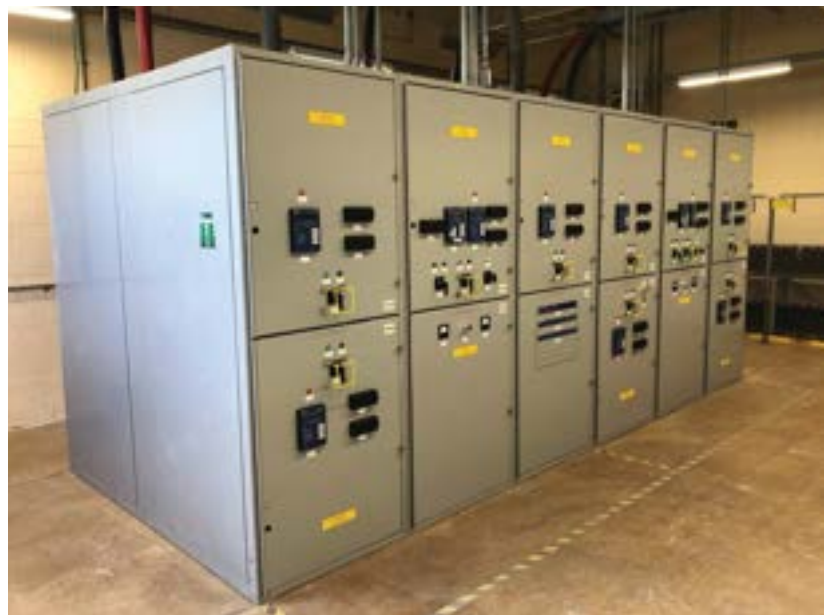
Figure 5: MV Switchgear after Relay Upgrade
