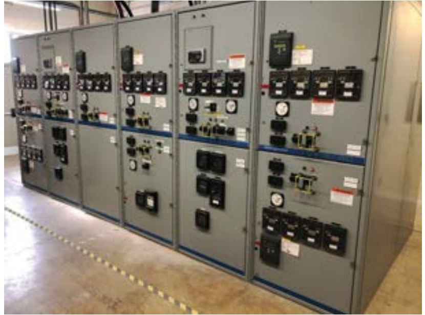
Figure 4: MV Switchgear before Relay Upgrade
