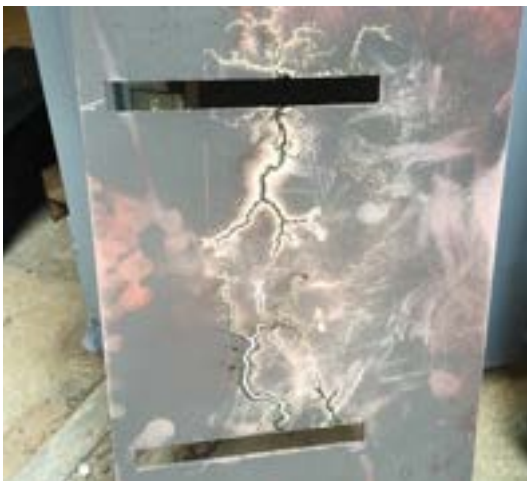
Figure 1: Tracking is an indication of insulation breakdown, which can lead to more significant failures.
