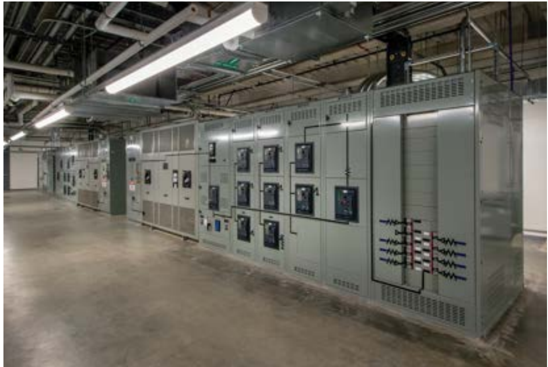
Electrical Room Control Panel
