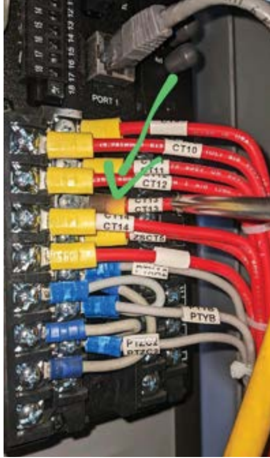
Figure 6: Overheating and Thermal damage at a CT Wiring Terminal
