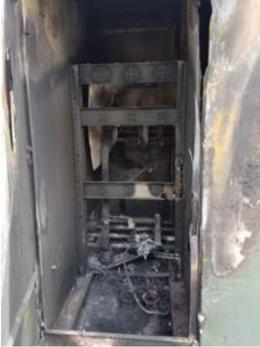
Result of a Sustained High Incident Energy Fault
