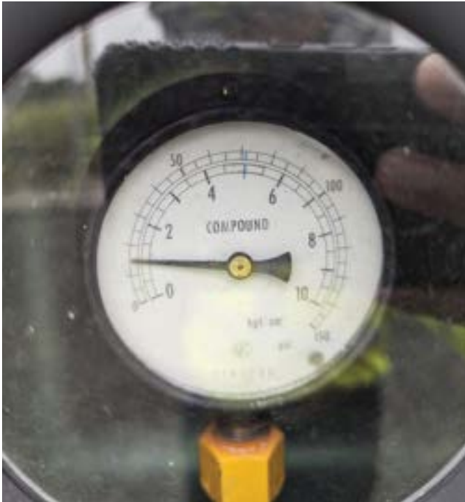
Figure 3: SF6 Pressure Gauge Reading on an Energized 121-kV Circuit Breaker
