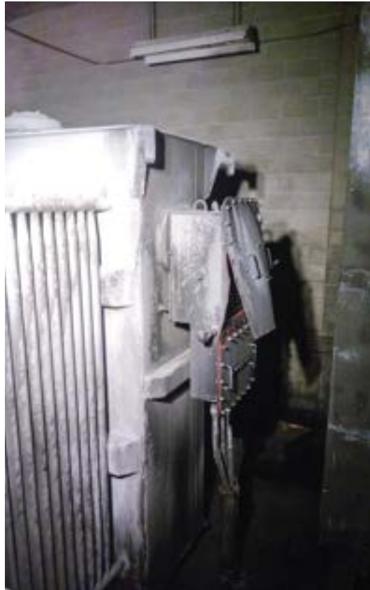
Result of a Low Incident Energy Flash in an Airtight Vessel
