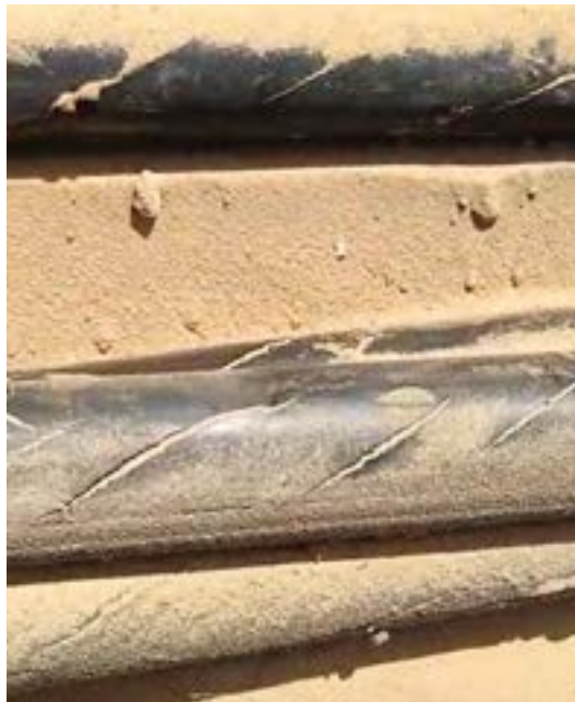
Figure 1: Damage Identified on the External Cable Jackets
