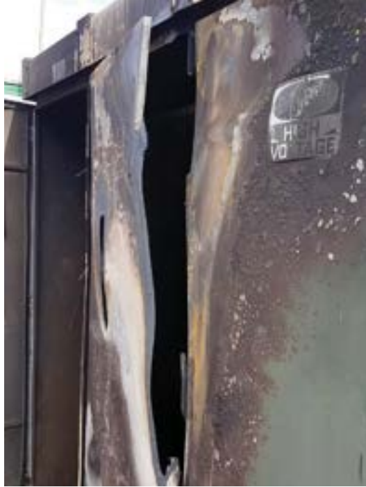
Auxiliary Damage Caused by High Incident Energy Fault
