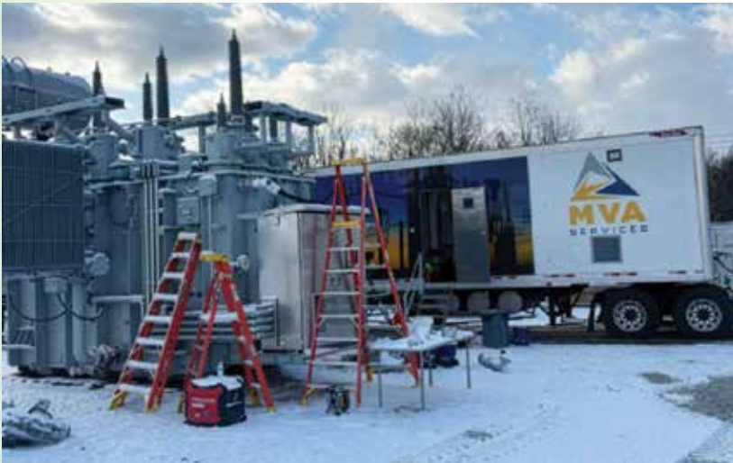
MVA at Work at a Transformer Project
