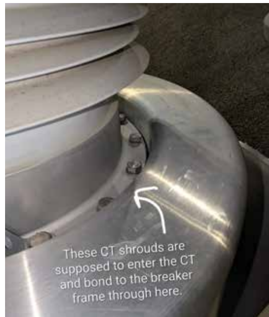
Figure 3a: Proper CT Shroud Bonding
