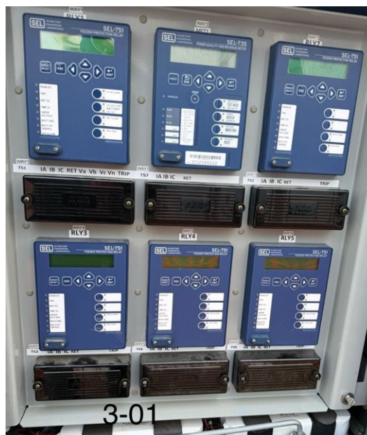
Photo 7: Protective Relays Using Fiber Outputs to Control the Automation
