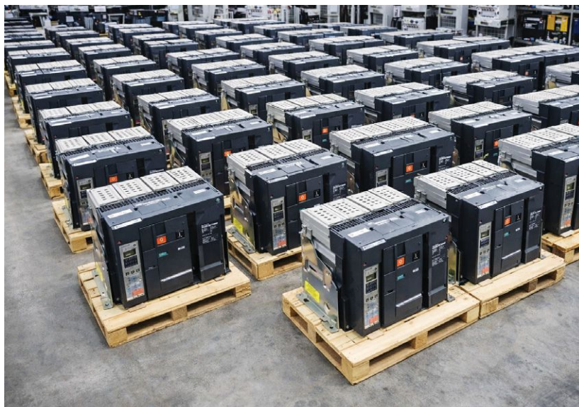
Photo 3: Low-Voltage Circuit Breakers in Just One Electrical Room
