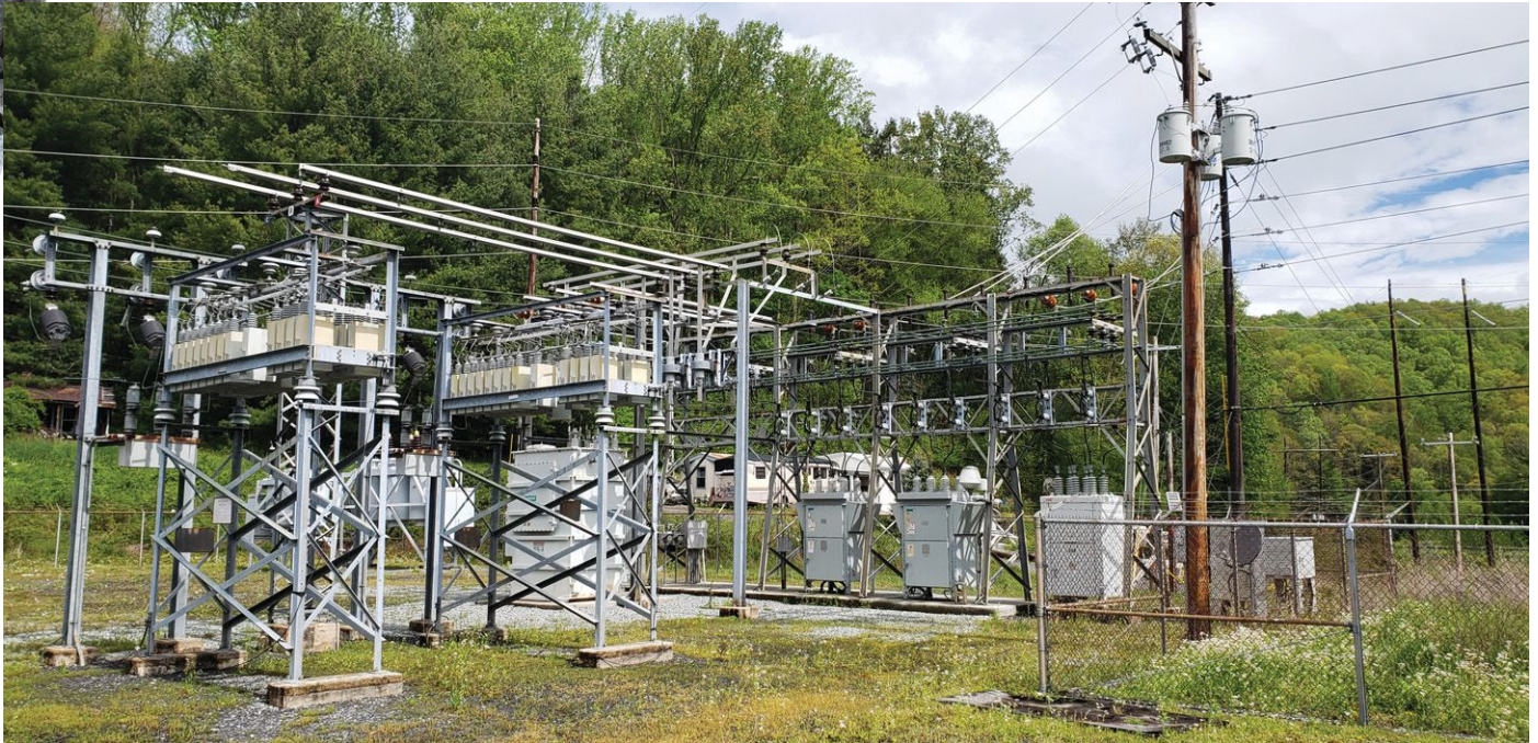
This older distribution substation has minimal rock with a lot of grass and weeds—precisely what you want to avoid.
