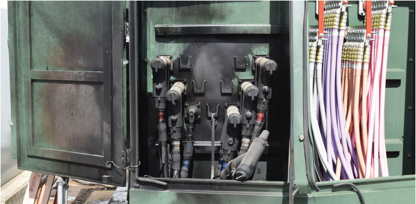
Photo 5: Transformer Fault Showing Internal Damage
