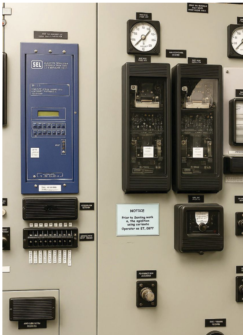
Figure 2: Existing Relaying Protection before Project Execution
