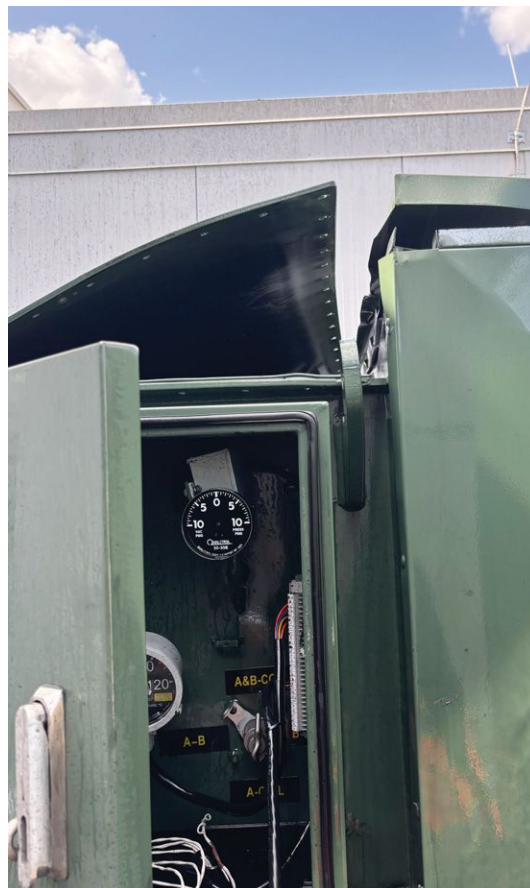
Photo 6: Equipment Damage from a Catastrophic Fault
