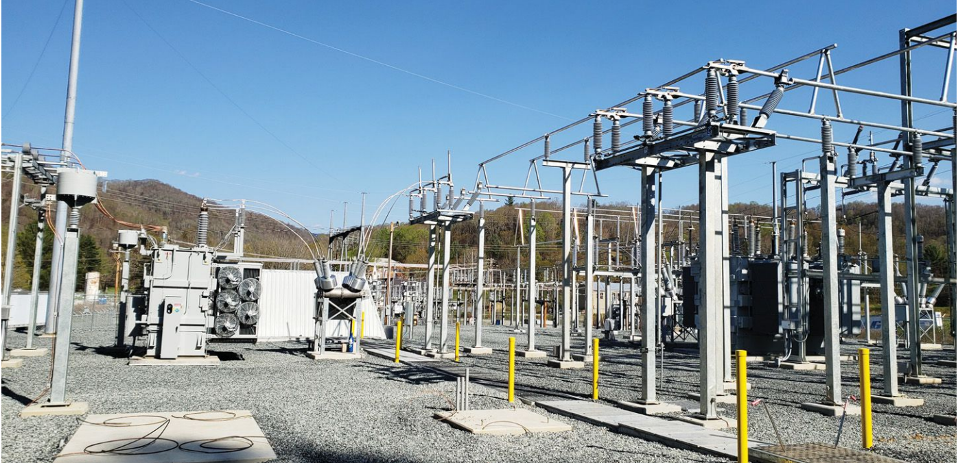
Regular inspections to maintain the rock layer depth are critical to substation safety.
