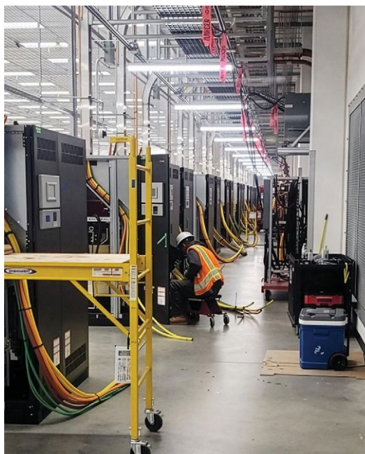
Photo 4: Numerous Power Distribution Units Installed in an Electrical Room
