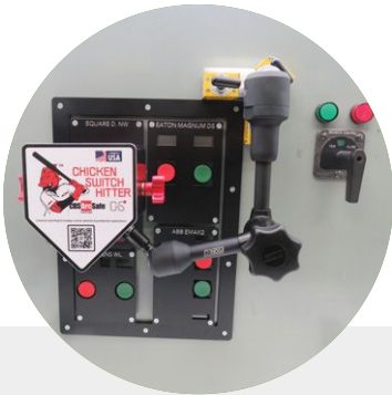
CBS Arc Safe — Arc-Safe Remote Racking Demo
