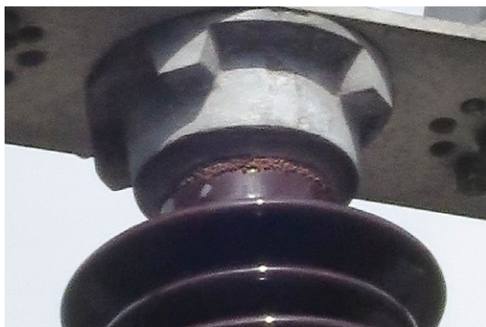
Figure 6: Visual Discovery of Corrosion on Insulator
